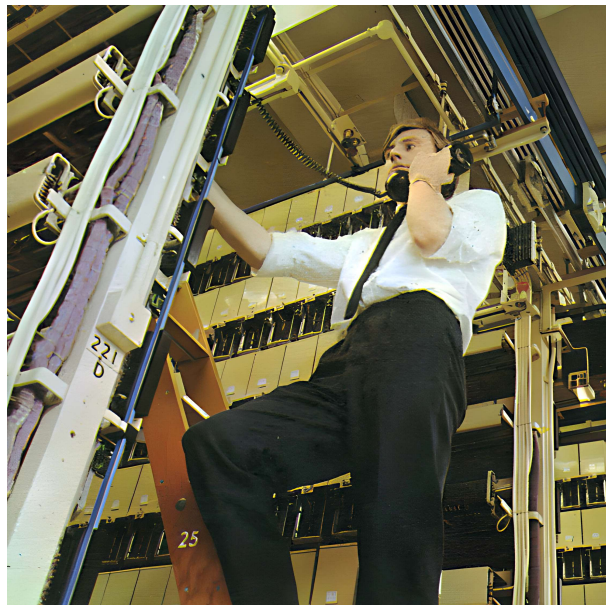
Technician working in a telephone exchange
