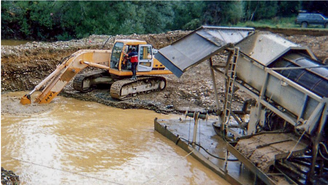
Graeme Hobb's floating gold recovery plant uses a rotating trommel screen. Fine material passes through the screen and falls on the sluice underneath. Oversized material exits at the end of the drum.
